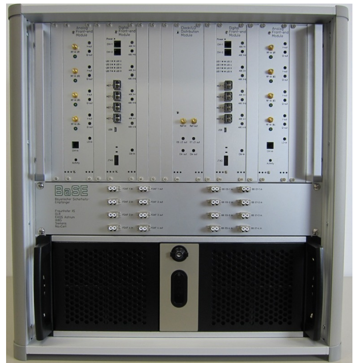
Figure 3: BaSE receiver setup without antenna
